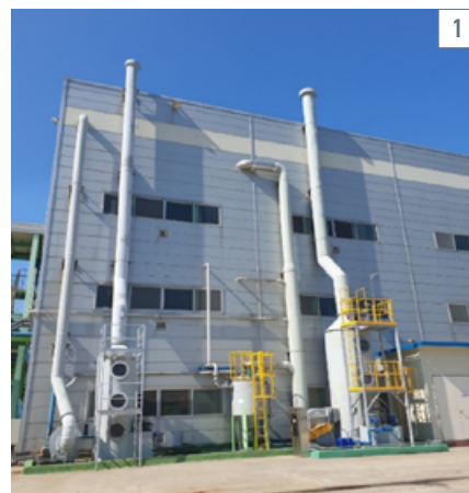
1. Air pollutant treatment facility (scrubber)
