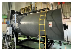
Low NOx boiler (10 tons)
