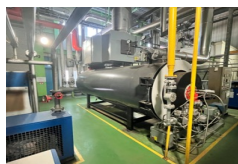
Low NOx boiler (3 tons)
